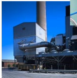
Opacity monitoring on a municipal waste incinerator
