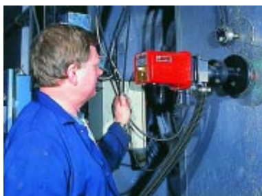
Dust monitoring on a coal-fired boiler
